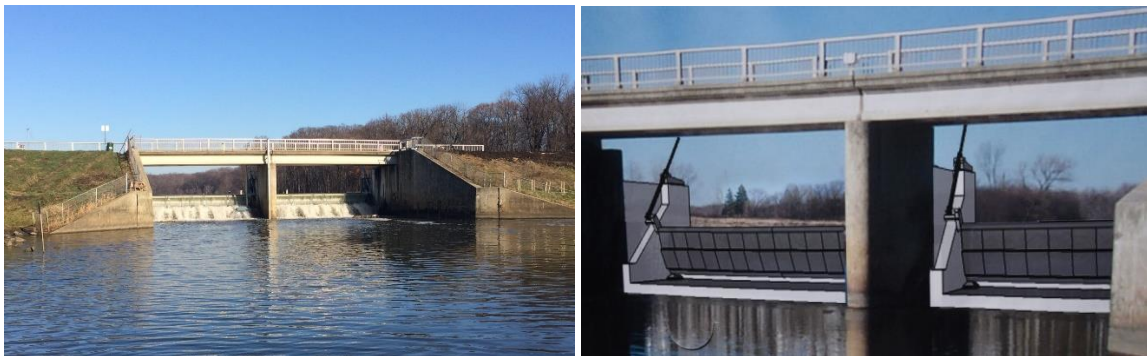
Completed modification of Busse Dam (left) and digital model of hinged gates (right).
