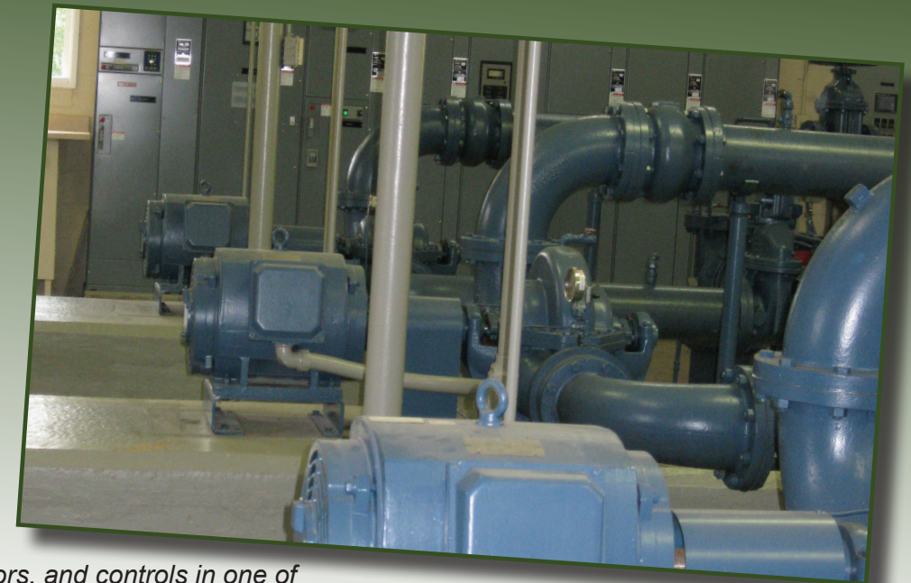
Pumps, motors, and controls in one of the Village's pumping stations.
