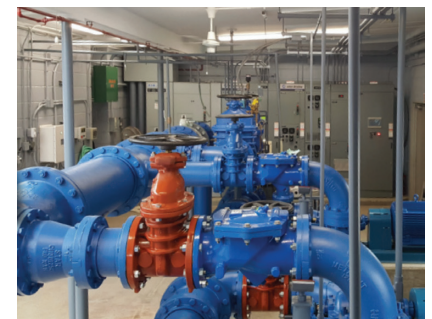
Pumps, motors, and piping in one of the Village's pumping stations. These pumping stations help deliver water to the community.
