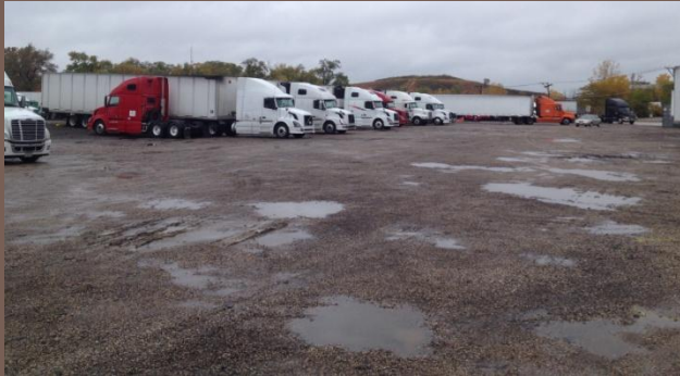
Deteriorated Parking Lots
