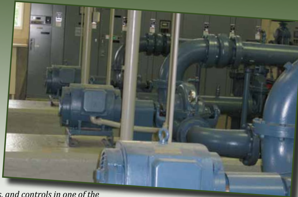
Pumps, motors, and controls in one of the Village's pumping stations.
