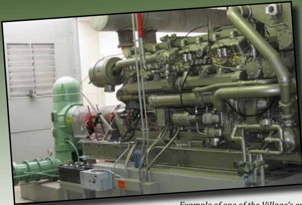
Example of one of the Village's emergency wells and the motor to power it.
